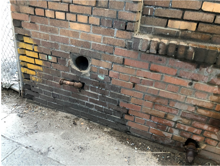
Photo 9: Vent pipe exiting 404 Exterior Street on the western side in north corner (facing east)
