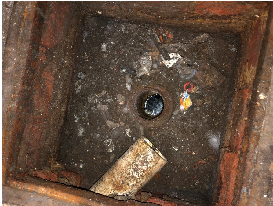
Photo 13: View of pit under metal plate in central portion of ground floor
