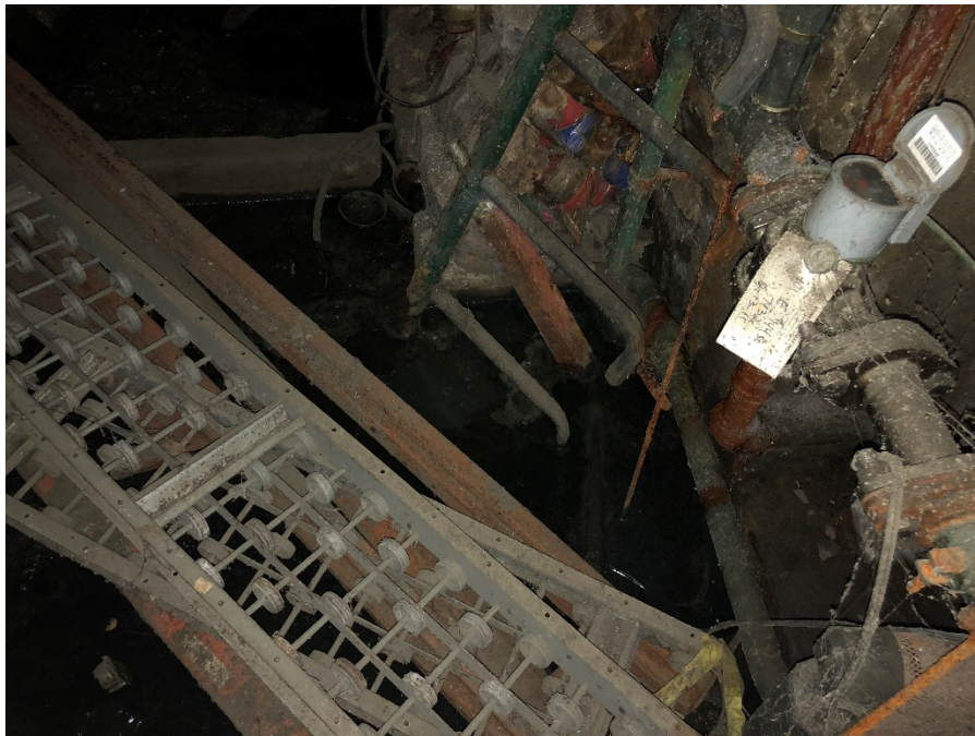
Photo 14: View of obstructions inside the northern cellar entrance and standing water on floor beneath
