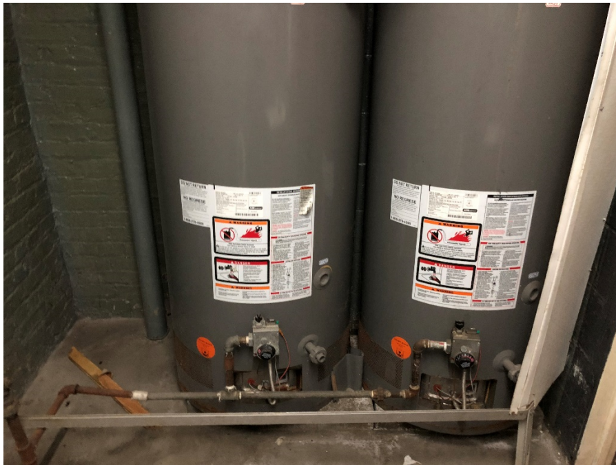
Photo 10: Water heaters in the northwestern part of the building (facing east)
