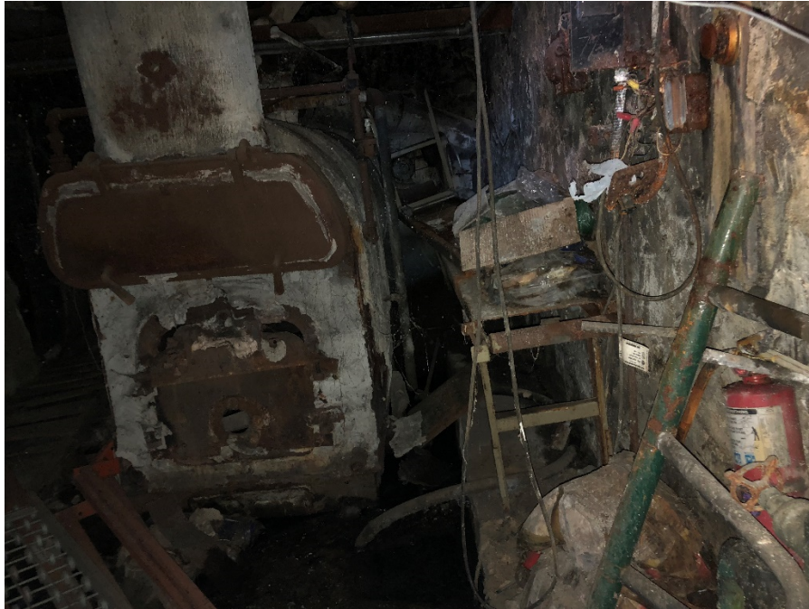
Photo 15: View of AST encased in concrete within the northern partial cellar (facing east)
