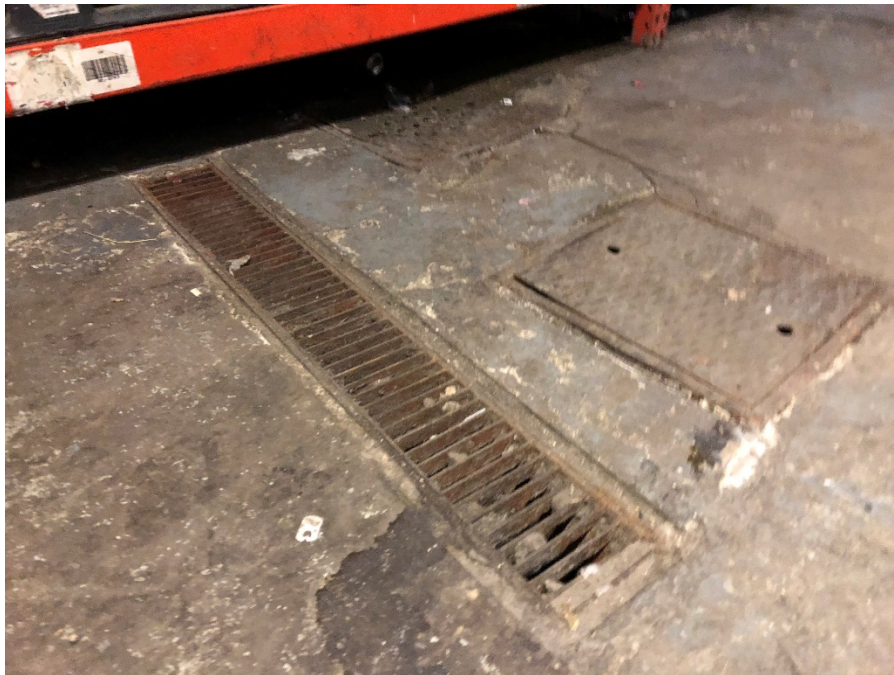
Photo 12: View of grated trench drain and two metal plate-covered pits within the concrete paved, central portion of the ground floor
