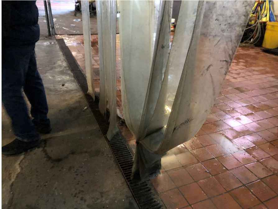
Photo 11: View of grated trench drain surrounding tiled food prep area (facing east)
